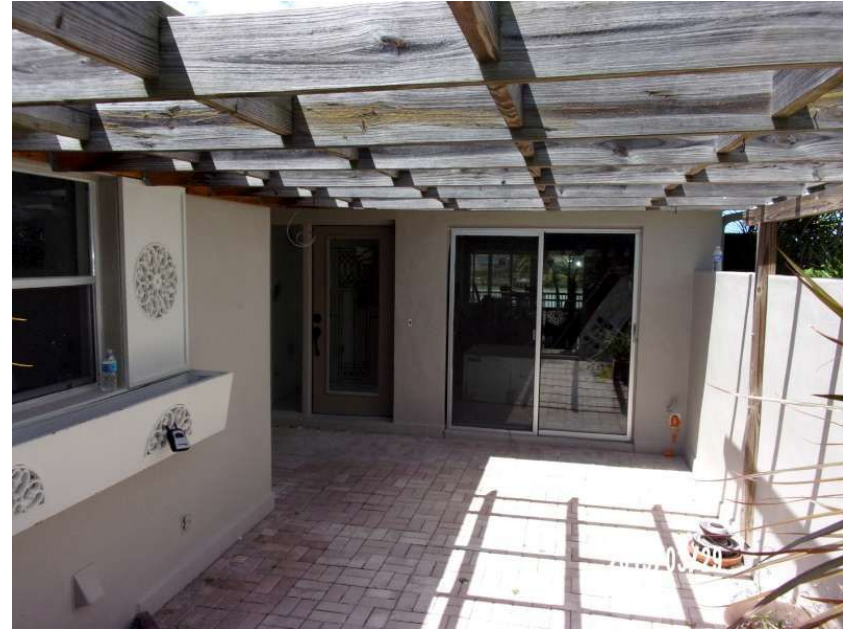
Unprotected Glazed Entry Door
