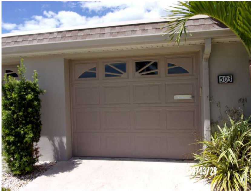
Unprotected Glazed Garage Door
