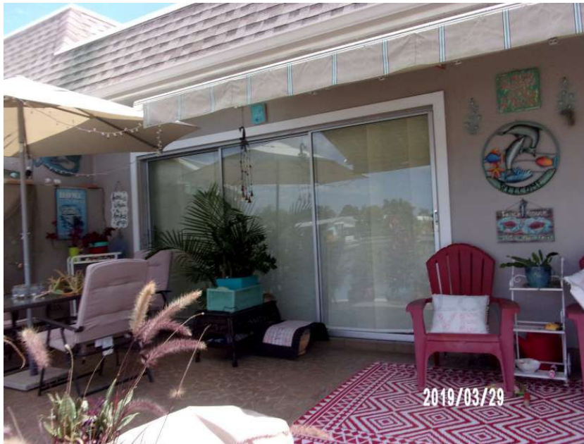
Unprotected Glazed Entry Door
