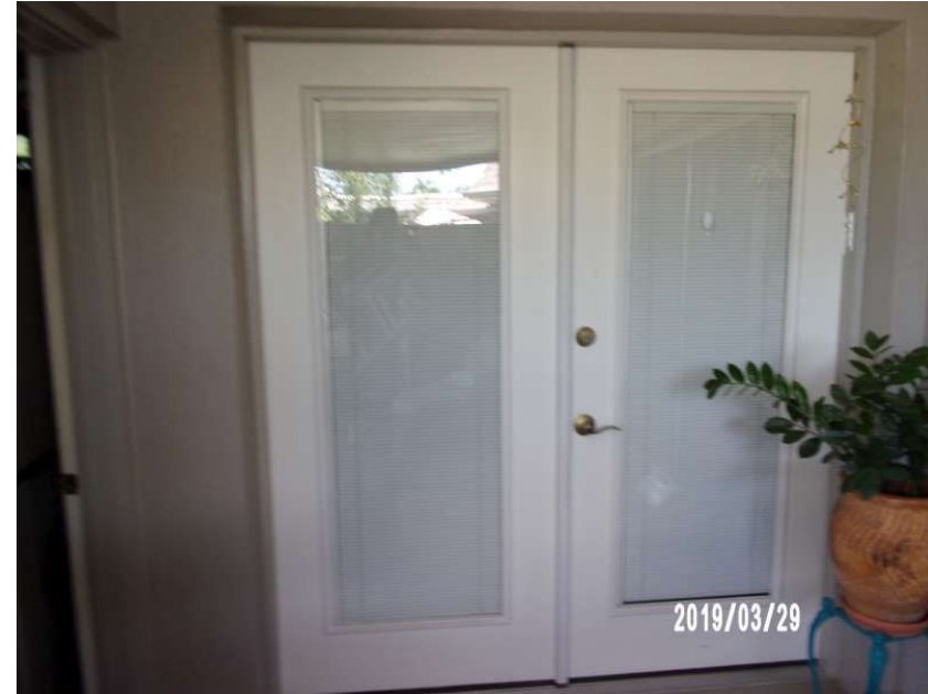
Unprotected Glazed Entry Door
