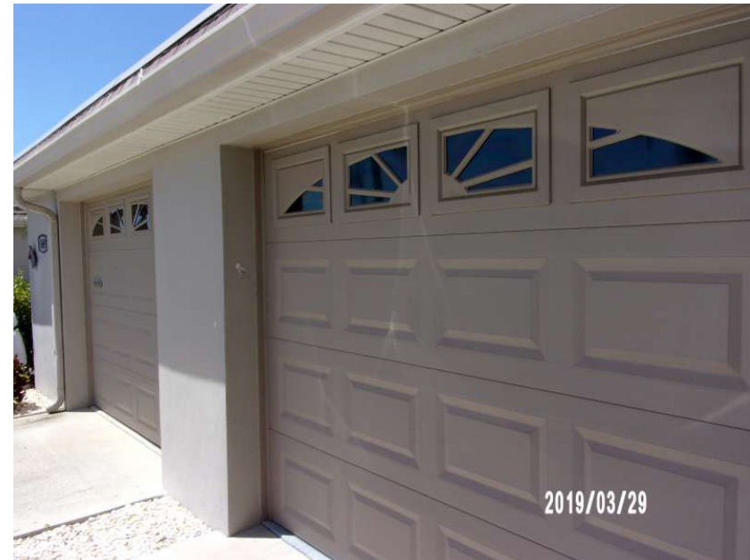
Unprotected Glazed Garage Door
