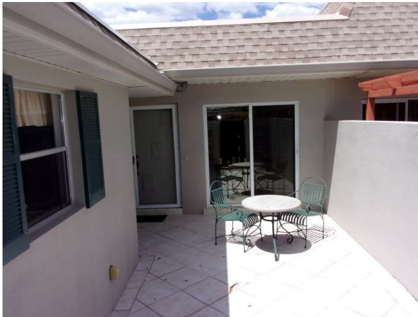
Unprotected Glazed Entry Door
